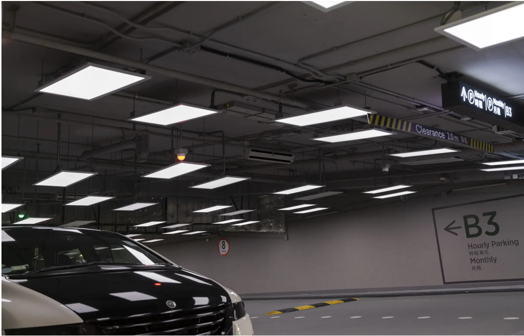
Light levels meet Building Code requirements; animated light sequences dim light levels to the code requirements but also to high intensities to add dynamism.
